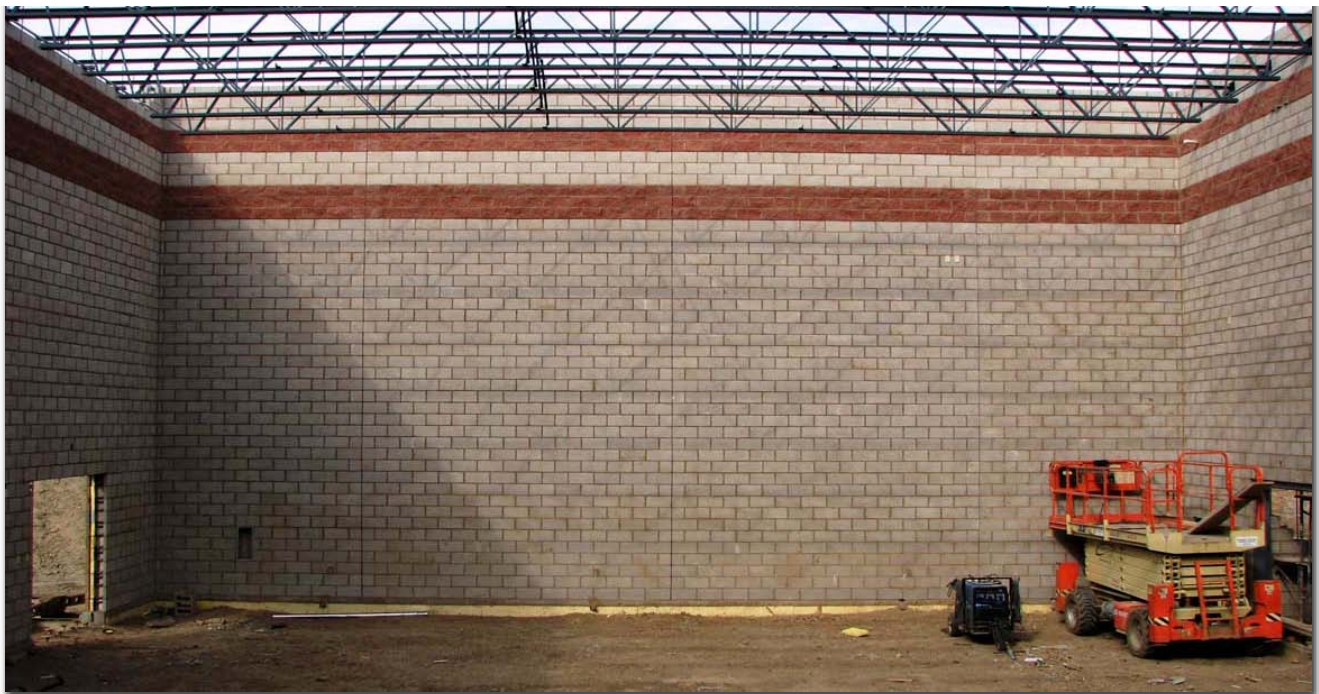
OneStep gymnasium, finished inside and out, completed in less than four weeks
